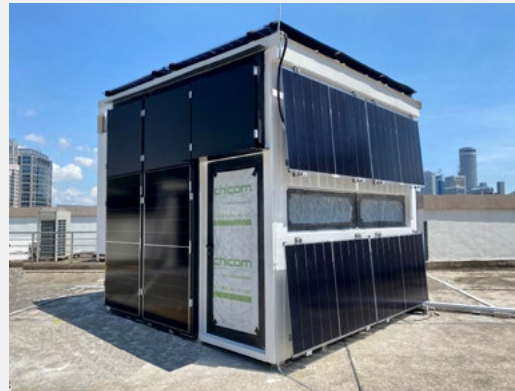
Diagram credit: SERIS, NUS Modular pod installed at Central Mall featuring modular BIPV blocks.
