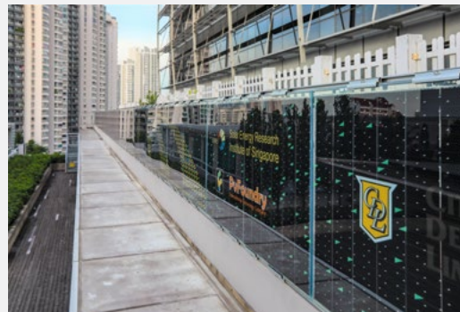
Bifacial BIPV printed panels piloted at City Square Mall.
